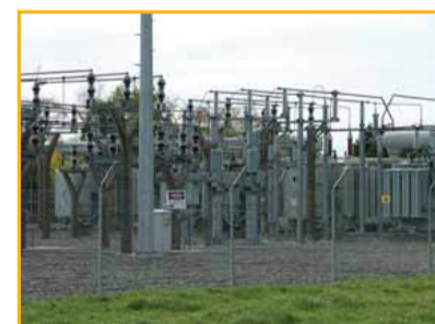
Transpower's Substation at Kaiapoi
